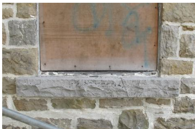
Allège no. 23, fissure
